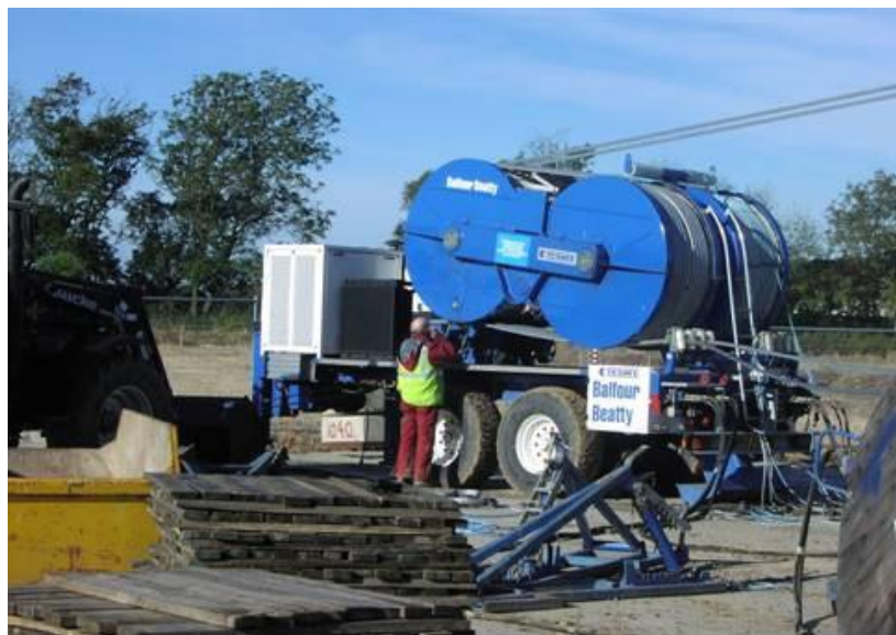
Photo B-6: Power Winch used for Pulling Wires along a Section of Overhead Line
