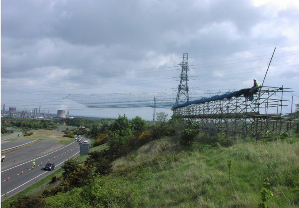
Photo B-7: Typical Scaffold and Netting to Safeguard Public Highway during Line Stringing (Fitting of Wires)
