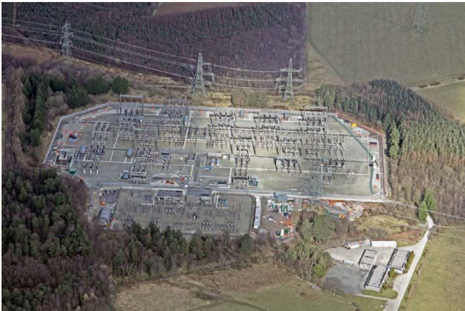
Photo Number 38. Detailed view of Pentir Substation. (11479-102).
